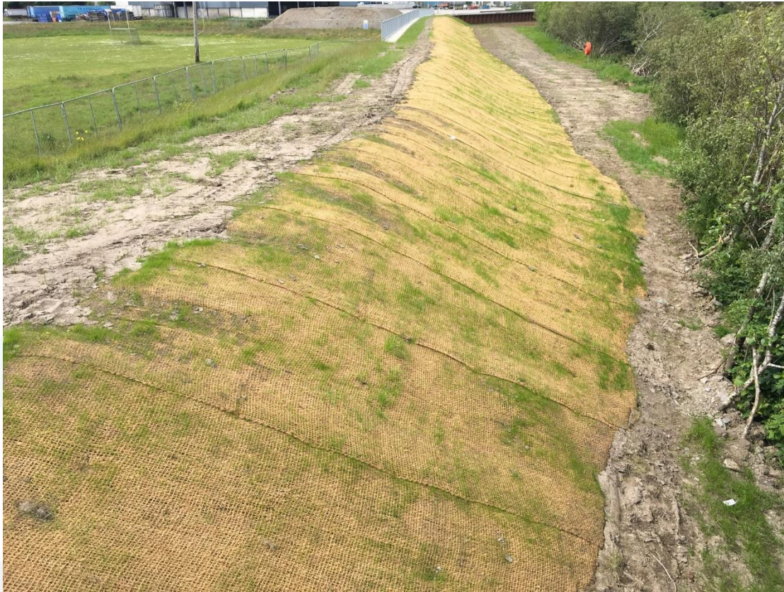
Plate 7 Large-scale use of CoriMesh to stabilise exposed ground, as likely required upstream of Wall 1 once large peat deposits are removed
